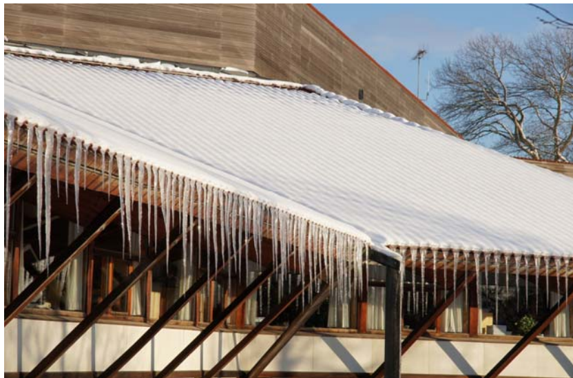
FIG 1. Icicles hanging from a building with large overhang
